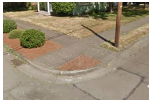
Intersection without Curb Ramps
